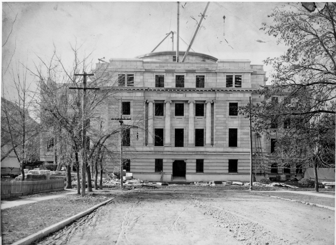
80-163.21-c Idaho State Capitol. View from side during construction of center part, dome not yet added.jpg
