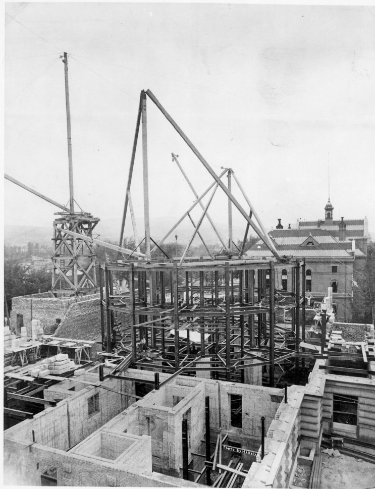
80-163.21-a Idaho State Capitol. Construction of first floor, framing begun for rotunda. 1906 or 1907.jpg
